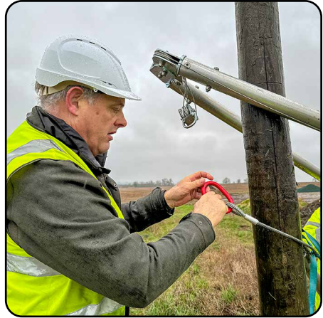
12. When the pole is up and back-filling is completed, slacken off the winch and when the shearlegs have been lowered to the ground the hitch on the pole will loosen itself and slide down. It can then be removed.
