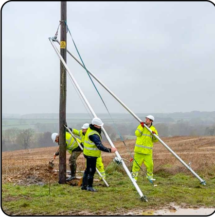
11. Use the shearlegs to hold the pole firmly in the required position during back-filling and tamping.
