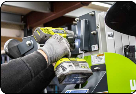
9. Use the impact wrench with 13mm socket to loosen all four nuts from the existing mast wire cover.
